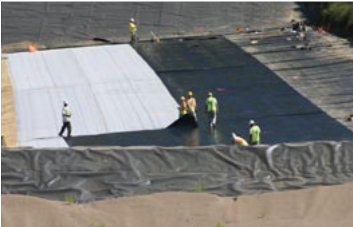
A composite liner system provides three layers of groundwater protection: two to four feet of clay, a geosynthetic clay liner and a geomembrane such as this being installed at the Alma Offsite.
